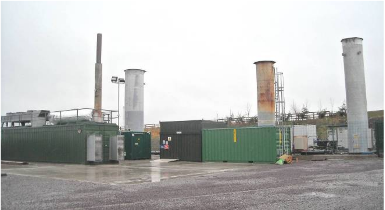
Plate 1-6: Landfill Gas Compound
